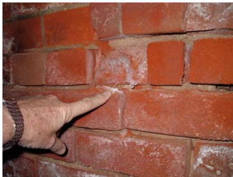
Figure 4 Salt crystal in basement wall - Royal Hotel Forbes
